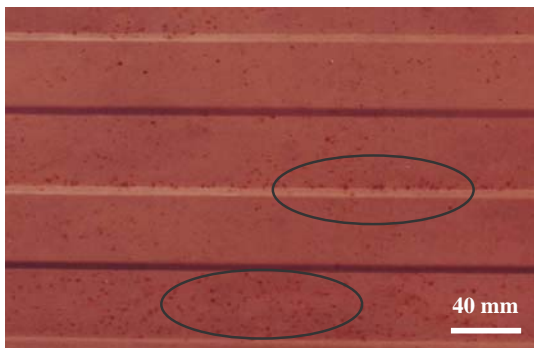
Figure 1: Red-brown rust spots (appeared as black spots) occurring on a panel.
