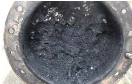
Fig. 7. Blocked Stripper Column due to Fouling
