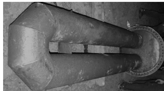
Fig. 8. Scale on Reboiler Fire tube
