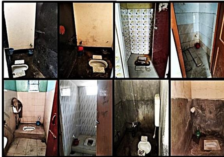
Figure 7 Images of sanitation facilities of different schools.
