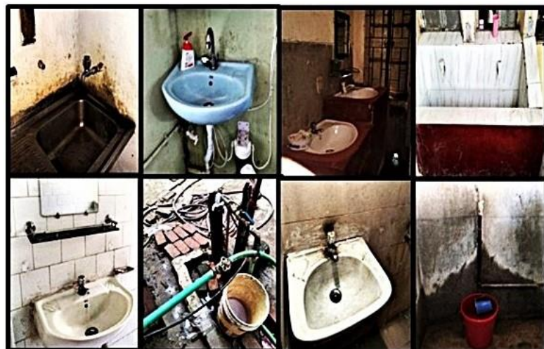
Figure 8 Images of hand washing facilities of different schools.
